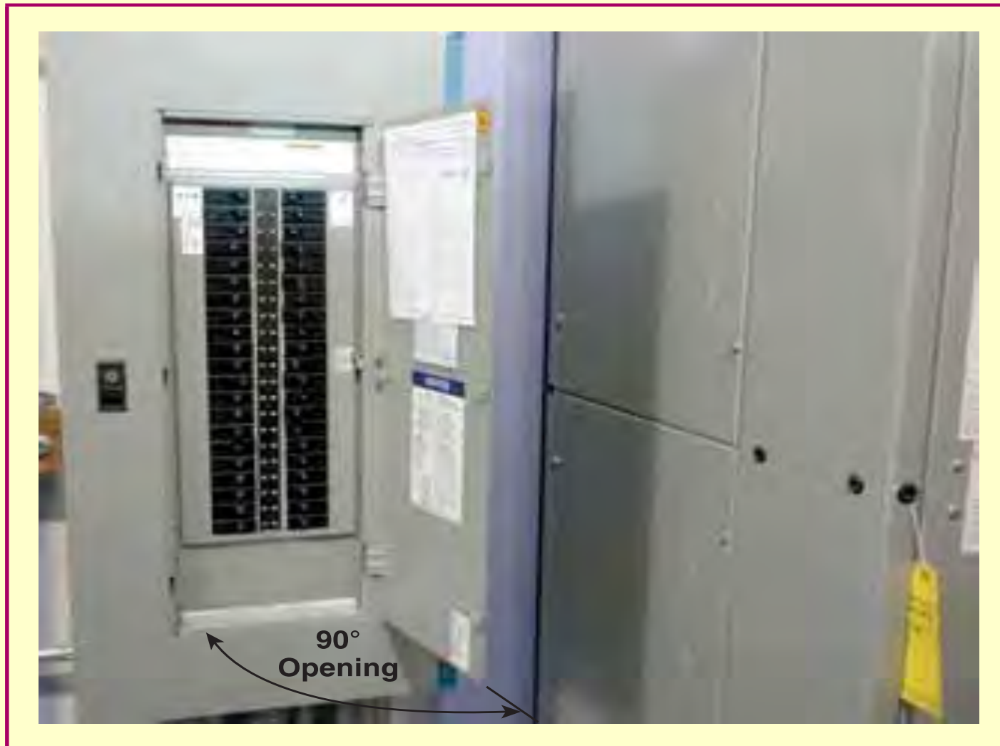
EXHIBIT 110.16 A full 90-degree opening of an equipment door in order to ensure a safe working approach.
