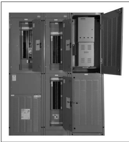
Figure 15. Integrated Facility System Switchboards
