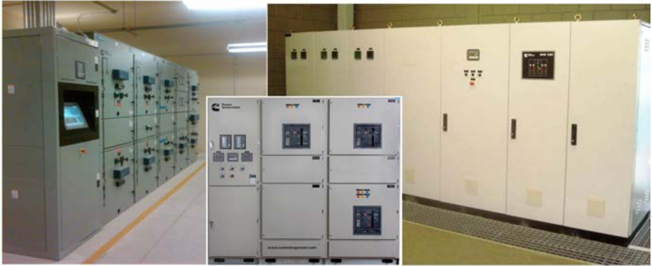
FIGURE 23. EXAMPLES OF SWITCHBOARD/SWITCHGEAR EQUIPMENT IN NORTH AMERICAN, SOUTH AMERICAN, AND IEC-BASED DESIGNS.
