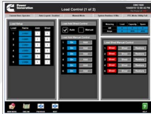
FIGURE 63. A TOUCHSCREEN INTERFACE PANEL THAT ALLOWS MANUAL CONTROL OF LOAD STEPS.
