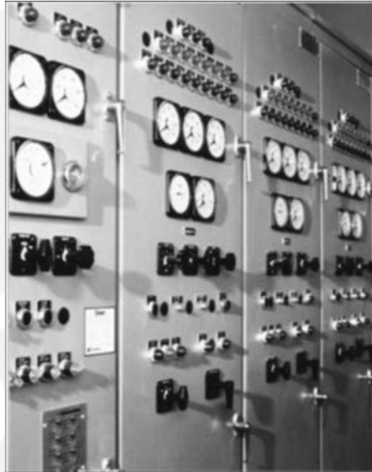
FIGURE 18. PARALLELING CONTROL PANELS WITH TRADITIONAL METERS AND SWITCHES.
