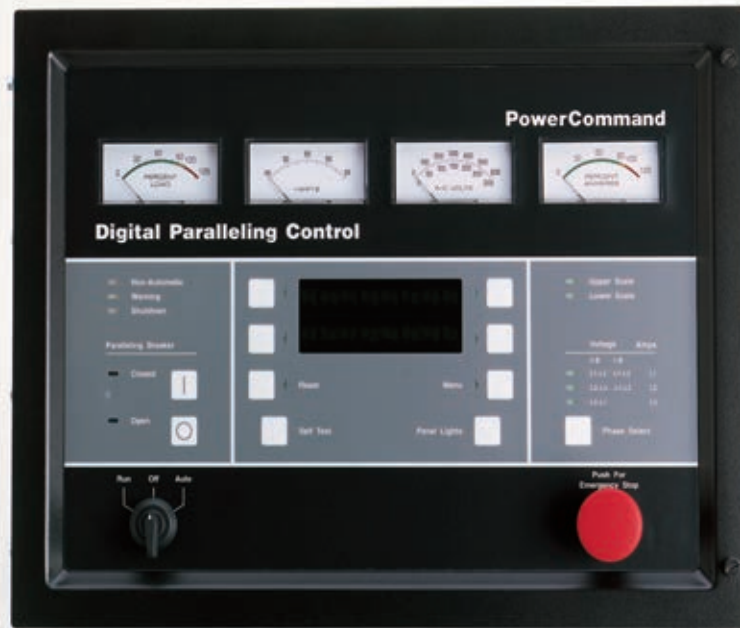
FIGURE 19. DIGITAL GENERATOR PARALLELING CONTROL. SIMILAR FUNCTIONS AS THE PARALLELING CONTROL SHOWN IN FIGURE 18 .
