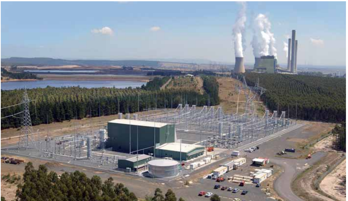
Fig. 2.5-18b, c: 400 kV HVDC Basslink project in Australia (monopole transmission line)
