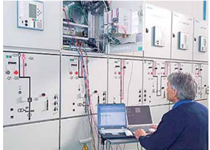
Fig. 6.2-25: Protection engineer at work
