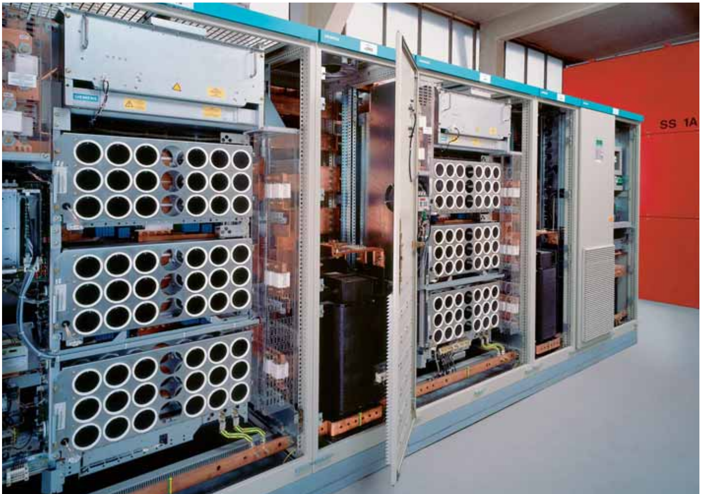
Fig. 2.3-1: SIPLINK with opened cabinet doors
