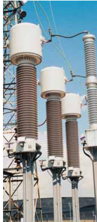
Fig. 4.5-1: 230 kV gas-insulated current transformers (on the left) and 230 kV oil-insulated capacitor voltage transformers (on the right)
