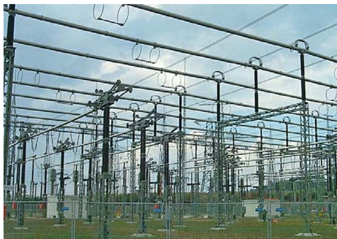
Fig. 3.1-20: Busbar disconnectors in diagonal arrangement, 380 kV, Germany
