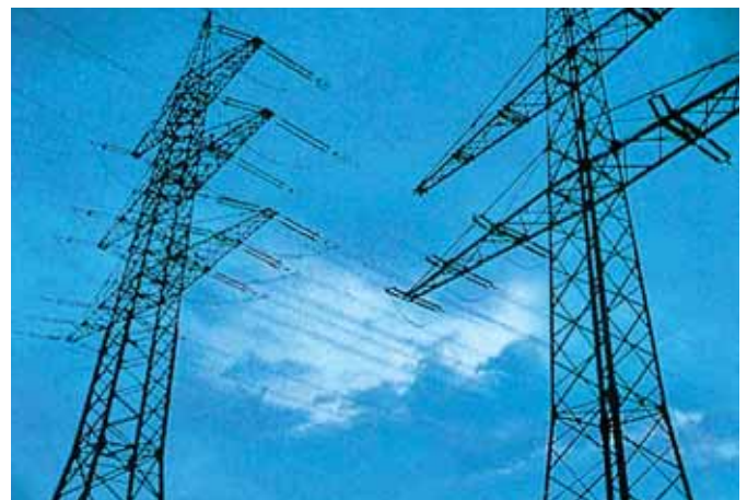
Fig. 6.4-19: ... and to monitor transmission lines
