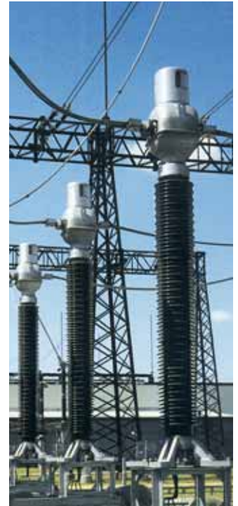
Fig. 4.5-2: 245 kV oil-immersed current transformers
