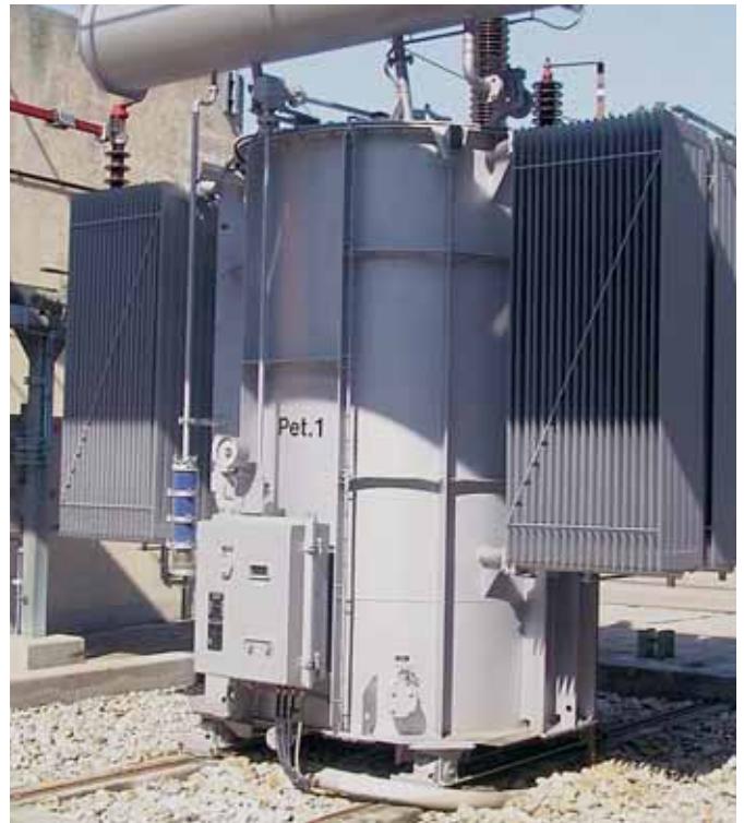
Fig. 4.6-5: Arc-suppression coil 110 kV
