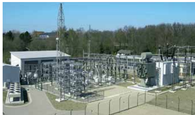
Fig. 2.4-2: Static Var Compensator (SVC) installation
