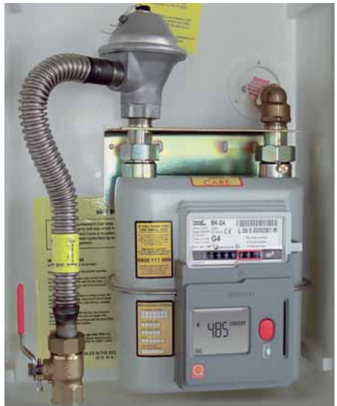
Fig. 10.3-3: Q-Smart prepayment meter installed
