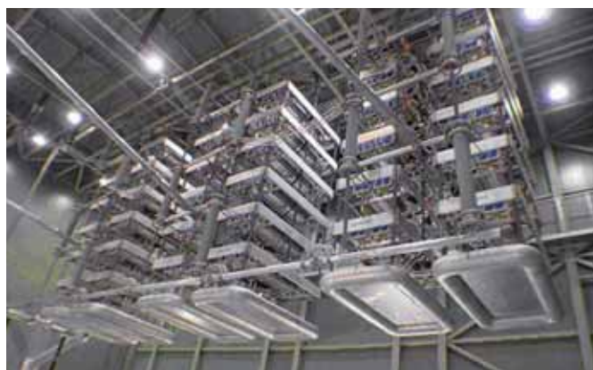
Fig. 2.2-2: Earthquake-proof and fire-retardant thyristor valves in long-distance transmission in Guizho-Guangdong, China
