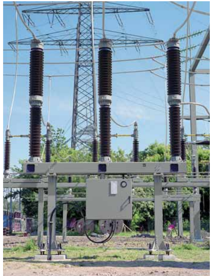
Fig. 4.1-9: 3AP1FG on site
