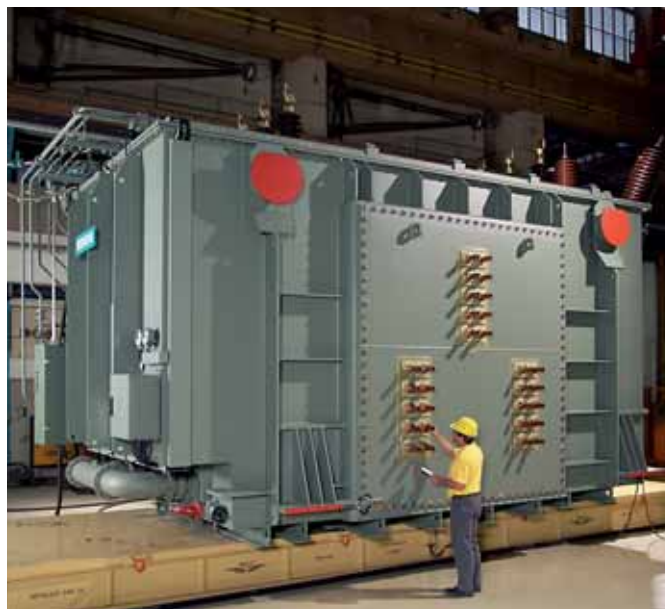
Fig. 5.6-1: Electric arc furnace transformer
