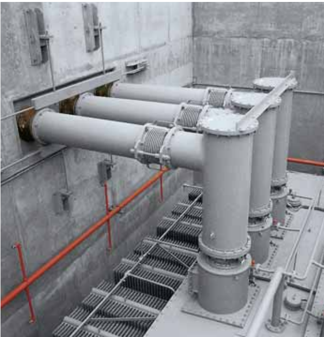
Fig. 3.1-48: Transformer termination modules
