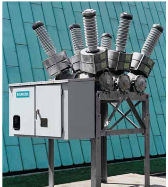
Fig. 4.1-11: SPS-2 circuit-breaker 72.5 kV
