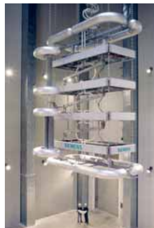
Fig. 2.2-5: UHV DC thyristor valve
