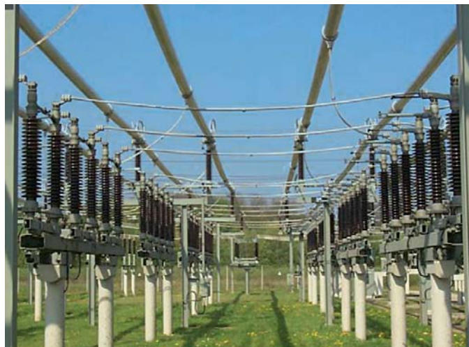
Fig. 3.1-16: Busbar disconnectors "in line", 110 kV, Germany
