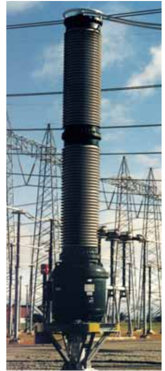
Fig. 4.5-5: 765 kV gas-insulated voltage transformer
