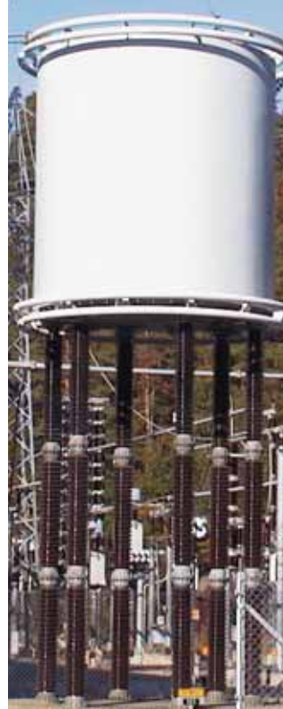
Fig. 4.6-4: HVDC smoothing reactor
