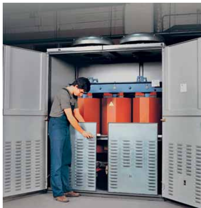
Fig. 5.9-8: GEAFOLE transformer in protective housing to IP20/40
