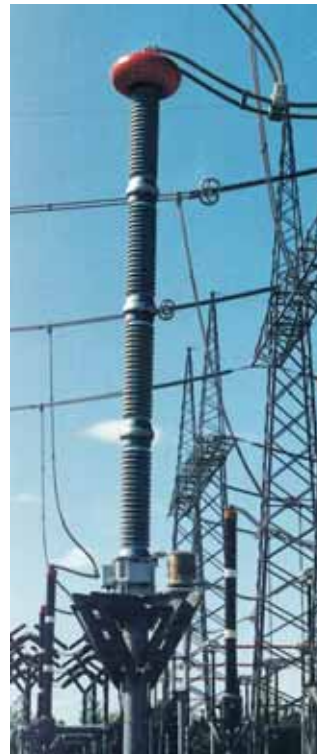
Fig. 4.5-6: 765 kV capacitor voltage transformer
