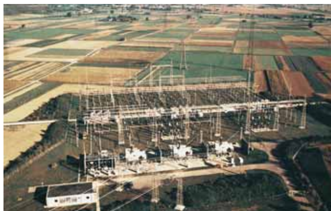
Fig. 3.1-2: Air-insulated outdoor switchgear
