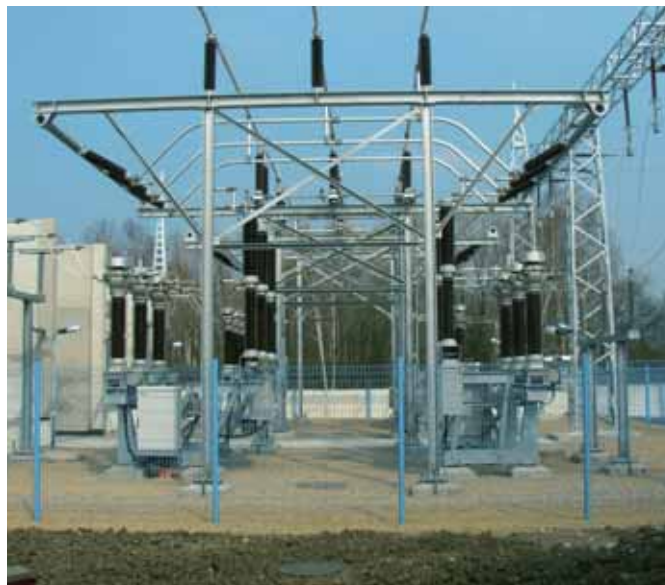
Fig. 3.1-30: H-arrangement with SIMOVER, 145 kV, Czech Republic
