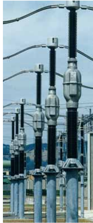
Fig. 4.5-4: 245 kV oil-immersed voltage transformer
