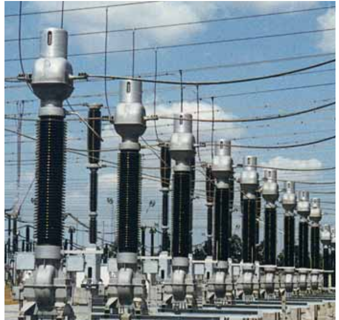
Fig. 4.5-8: 245 kV oil-immersed combined instrument transformer
