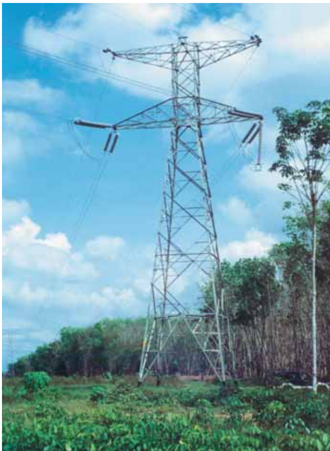
Fig. 2.5-17: 300kV HVDC interconnector from Thailand to Malaysia (bipole transmission line)
