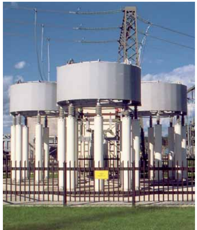
Fig. 4.6-3: Tertiary-connected shunt reactors
