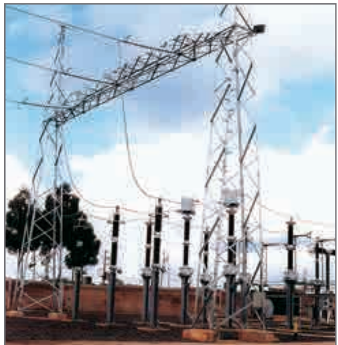
Figure D2.4: Carrier coupling equipment
