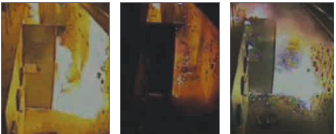
Figure C11.5a, 5b, 5c: Light arcing flash
