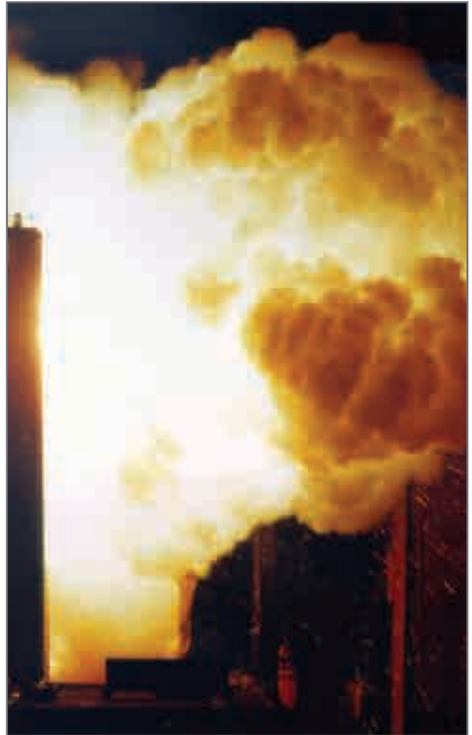
Figure C11.3: [Photo: J.Vogler]: Electrical explosions as result of an arc fault
