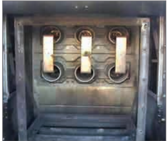
Figure C11.2a: Arcing time 47ms - Minor damage
