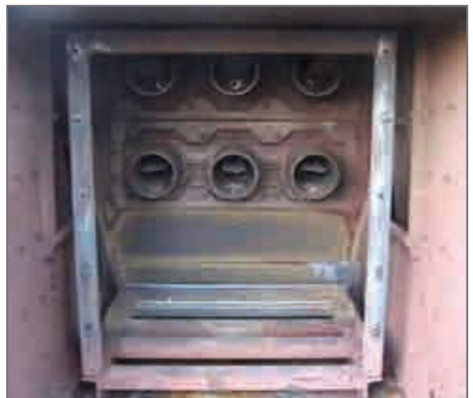
Figure C11.2b: Arcing time 500 ms - Copper busbars have evaporated
