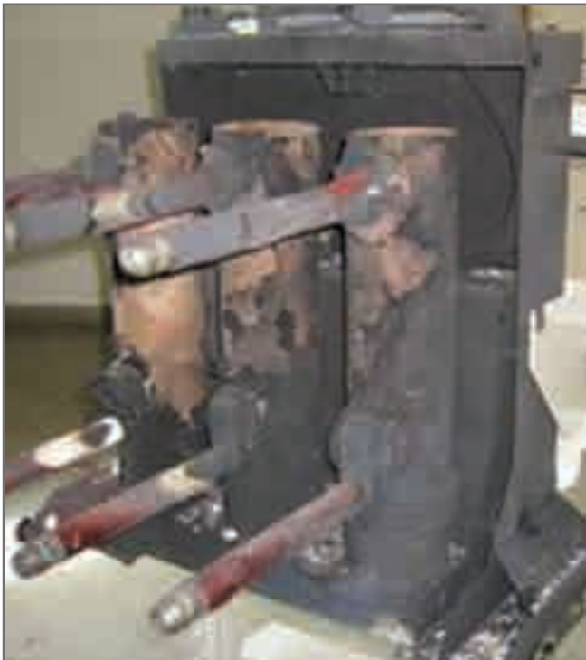
Figure C11.6a: Damage after an arc fault
