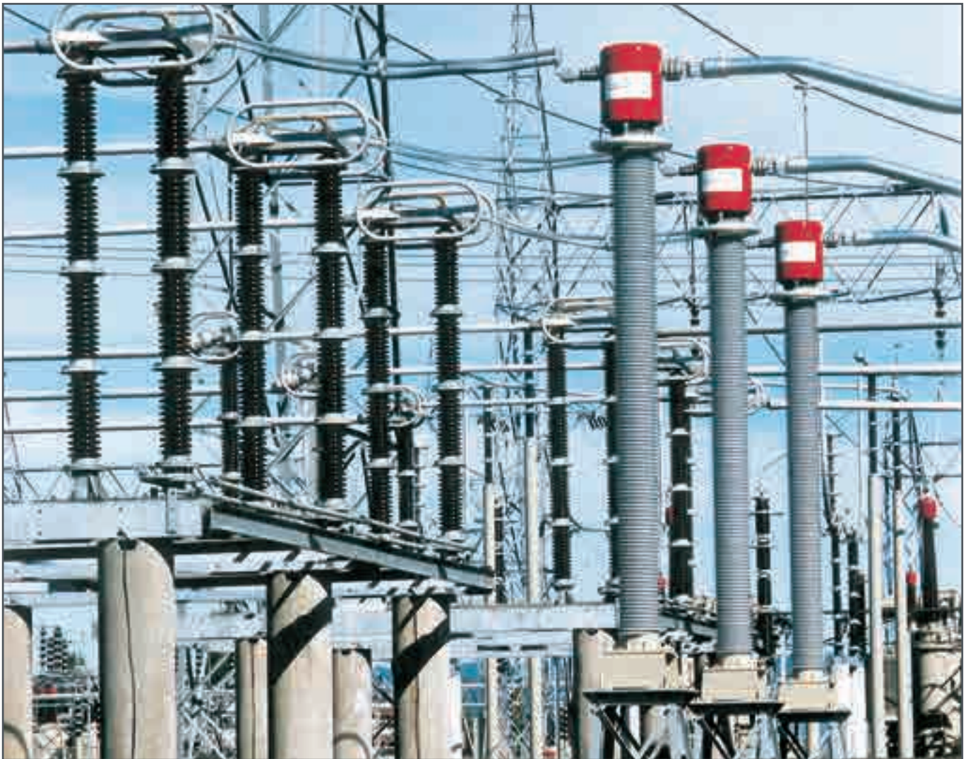
Figure B2.24: Field installation of a combined optical CT/VT
