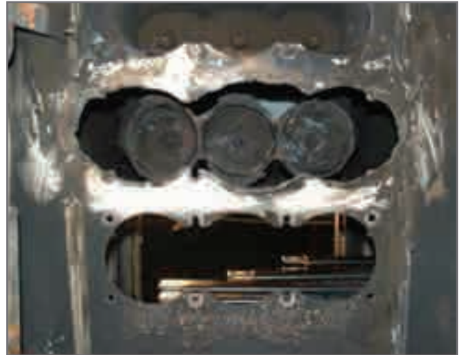
Figure C11.6b: Damage after an arc fault
